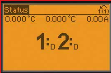
Read the compressor status directly from the display. D = Variable speed control, O = Off, R = Mains operation, X = Deactivated
