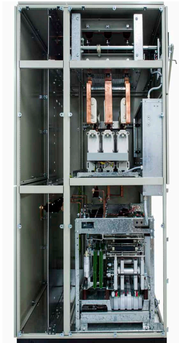
Side view of MVS panel with panels removed.
