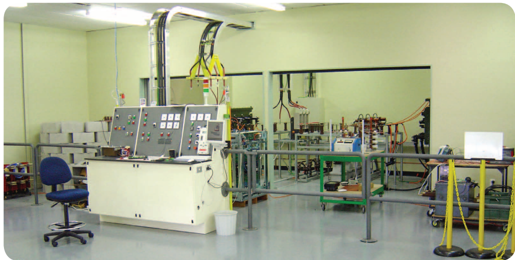
AuCom's medium voltage testing facility
